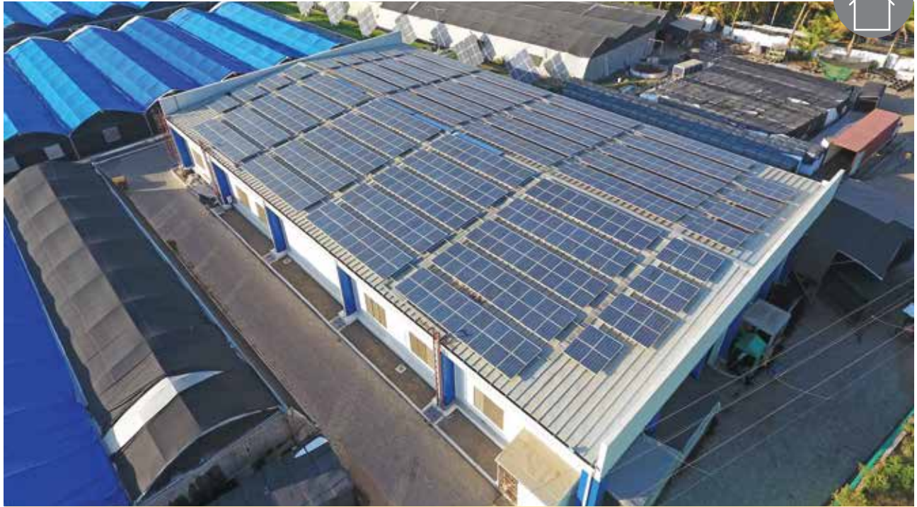
Solar Roof Top Grid Connected Plant
