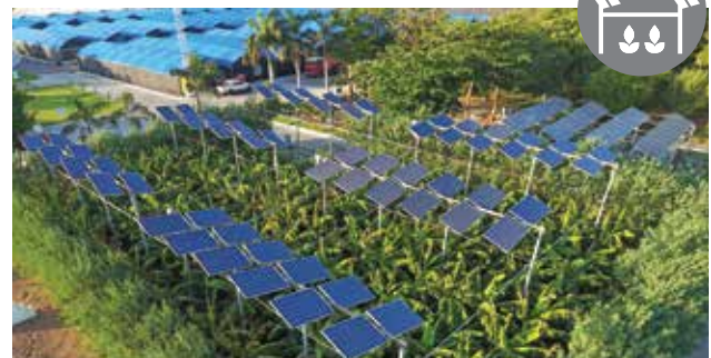
Solar AgroVoltaic Plant
